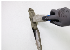
Close the damaged area discreetly.
